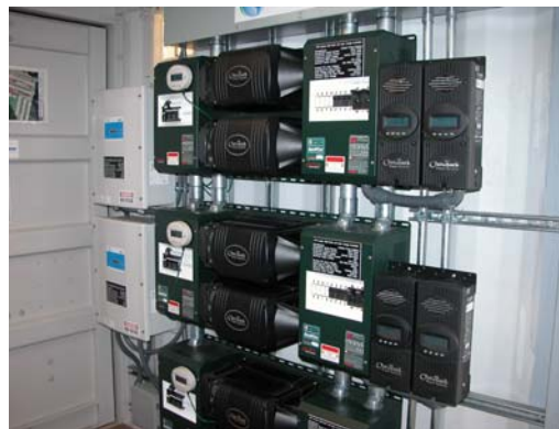
Inverters to convert DC power to AC power
